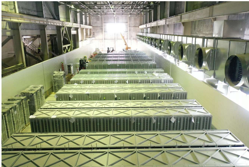
23 Battery packs inside Phase I of Moss Landing BESS. Credit: LG Energy Solution
